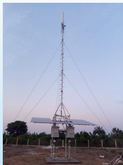
All-on-pole site @ Nigeria
