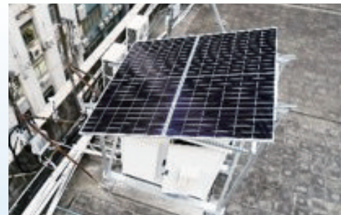
Solar on cabinet
