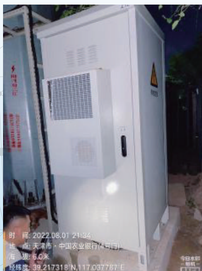
All-in-one cabinet site @ China Mobile
